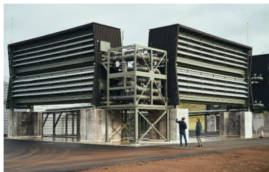
Fig. 1. Picture of Climeworks Orca plant running since 2021 in Iceland
